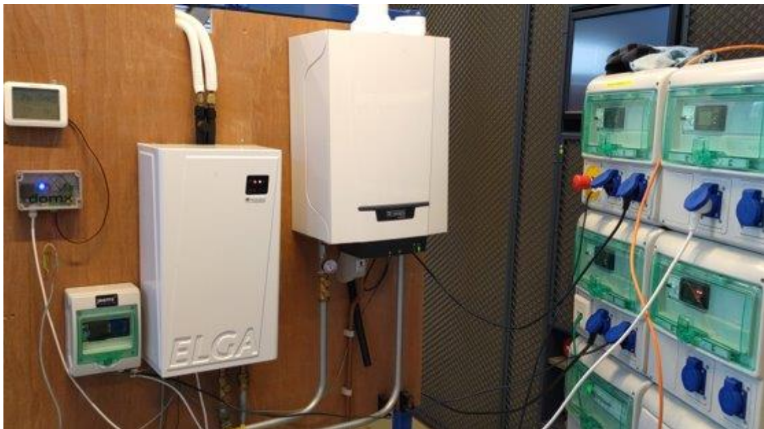
Figure 4: The hybrid heat pump setup in the HESI lab (Elga heat pump on the left and gas boiler on the right)
